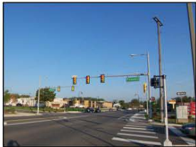
A. Traffic signals mounted on mast-arms
